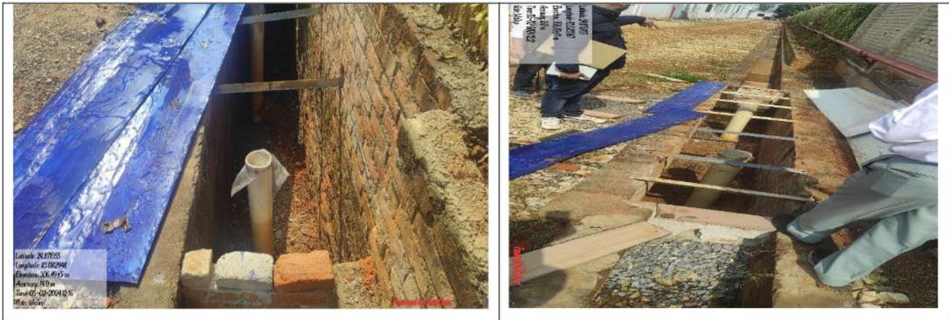
Photo -03: Rain water harvesting pits
