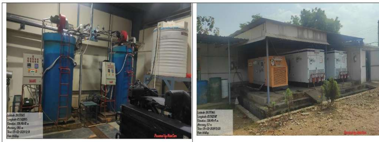
Photo -04: Gas Boiler and DG Sets
