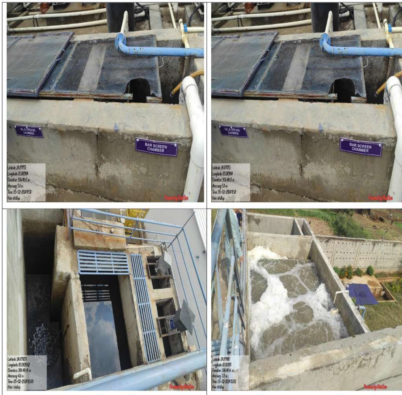
Photo -02: Effluent Treatment Plant of the Unit
